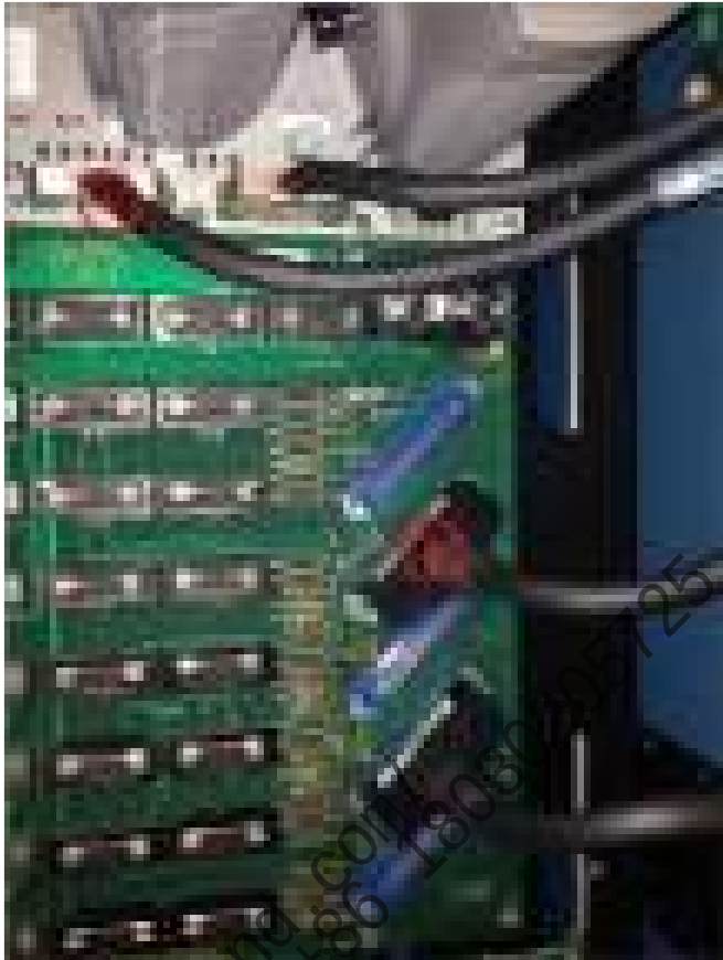
Figure 137: New cable connected from UHIO IOTA to TCBs
